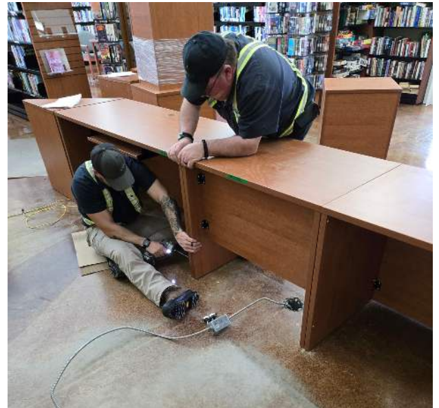
Adrien LeBlanc (sitting) and Barry Faulkner (standing) as they assemble the desk in Weymouth. Both are employees of the Municipality of Digby.
